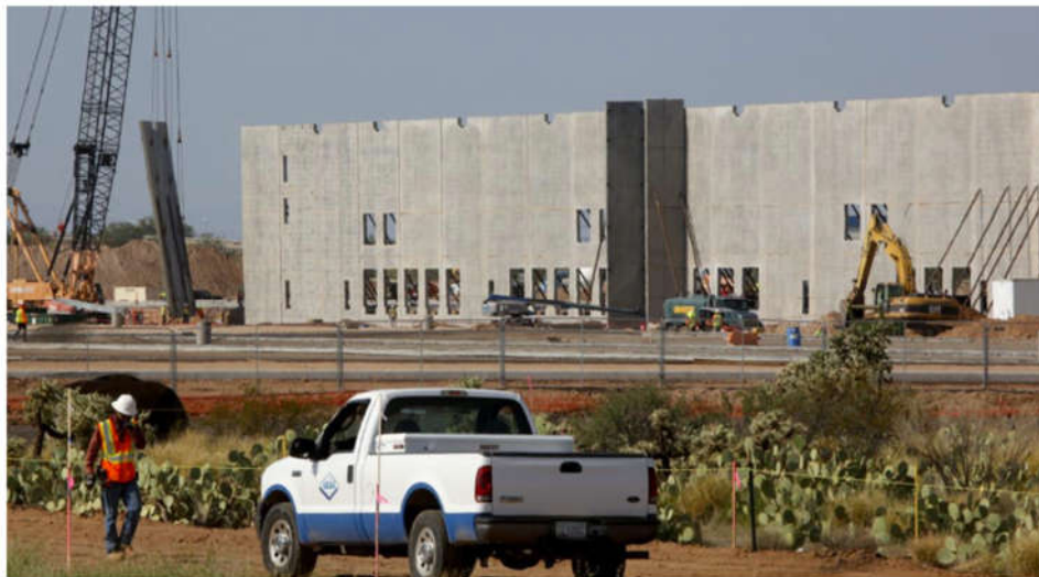
A section of wall goes up at what will be an Amazon warehouse and distribution center at South Kolb and East Valencia roads. The facility, which will employ about 1,500 Tucson workers, is expected to begin operations by the summer of 2019.
